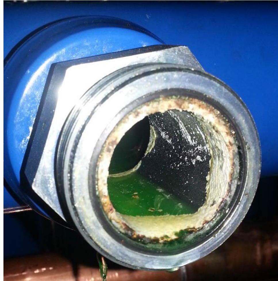
Zinc plated fitting with "white rust" on a spray ring manifold. Zinc is incompatible with Sunapee's process liquid. – 6 Nov 2013
