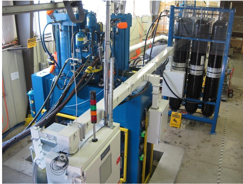
Figure 8: 40 kW Pilot unit at the original Lebanon, NH location, showing cylinders and air storage vessels (back right)
